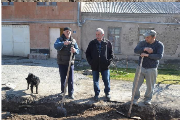
The community took over the trenchwork. On the photo, the residents helping to backfill the trenches.
