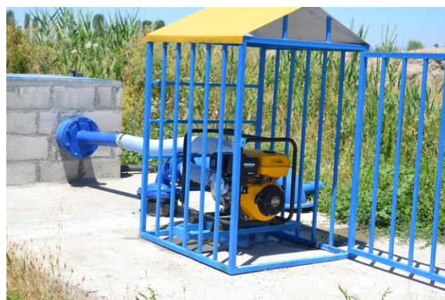
The booster pump installed in Sipanik.
