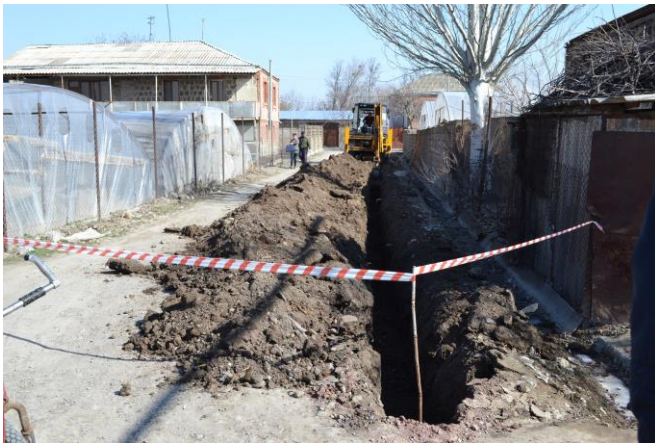
Drinking water pipework in Aratashen community.
